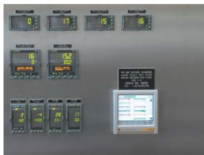
APV control panel
