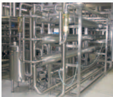
RO (Reverse Osmosis)
